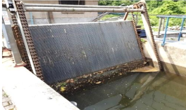
Figure 6. Intake screen near small hydropower plant [5].
