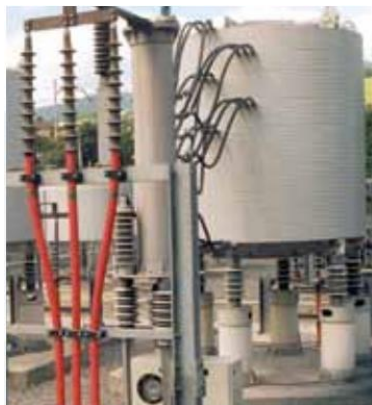
Figure 2. Air core tapped reactor (with 5 taps)
